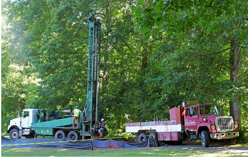
New Irrigation Well
