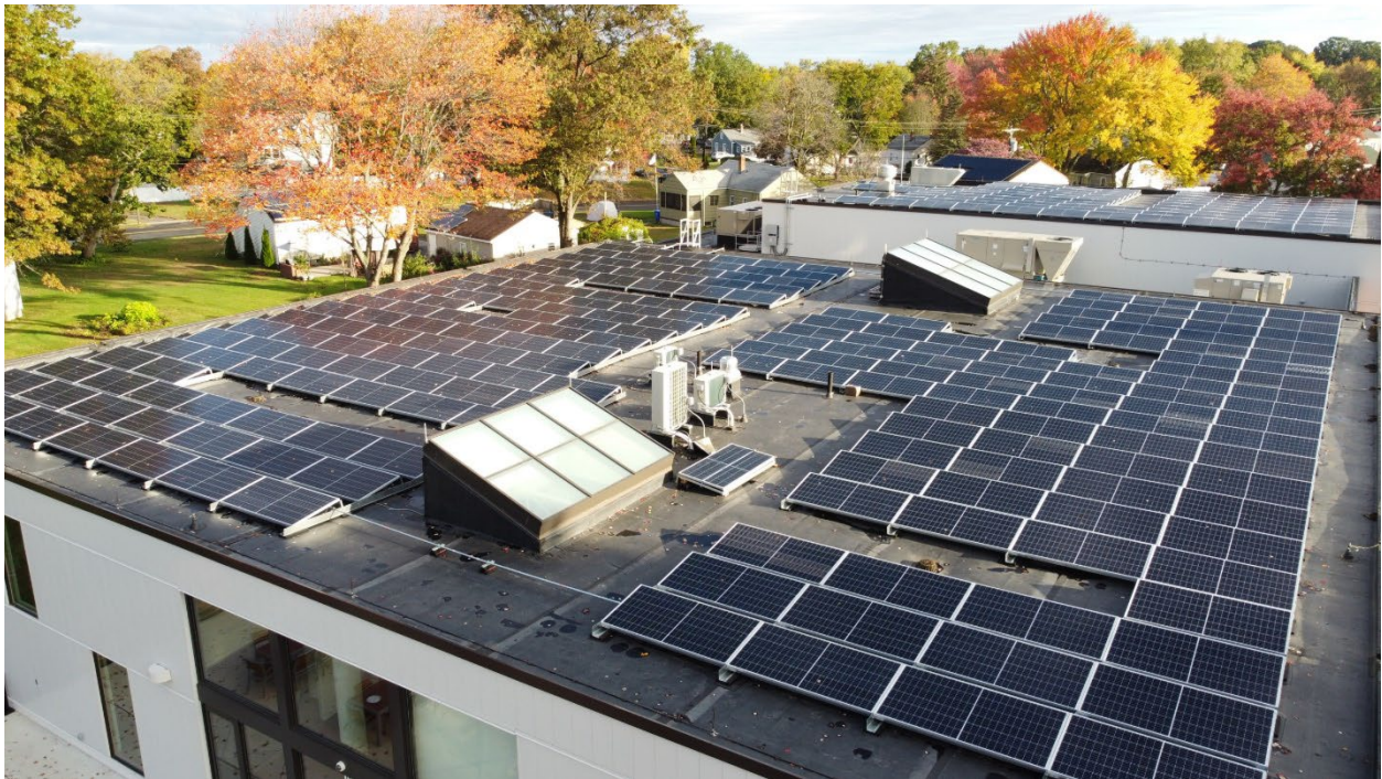
121 kW Solar Array on the Roof of the East Hartford Senior Center. Image Credit: Verogy
