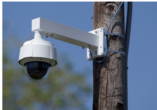
Above: A pole mounted camera gives police staff video of real-time traffic conditions.
