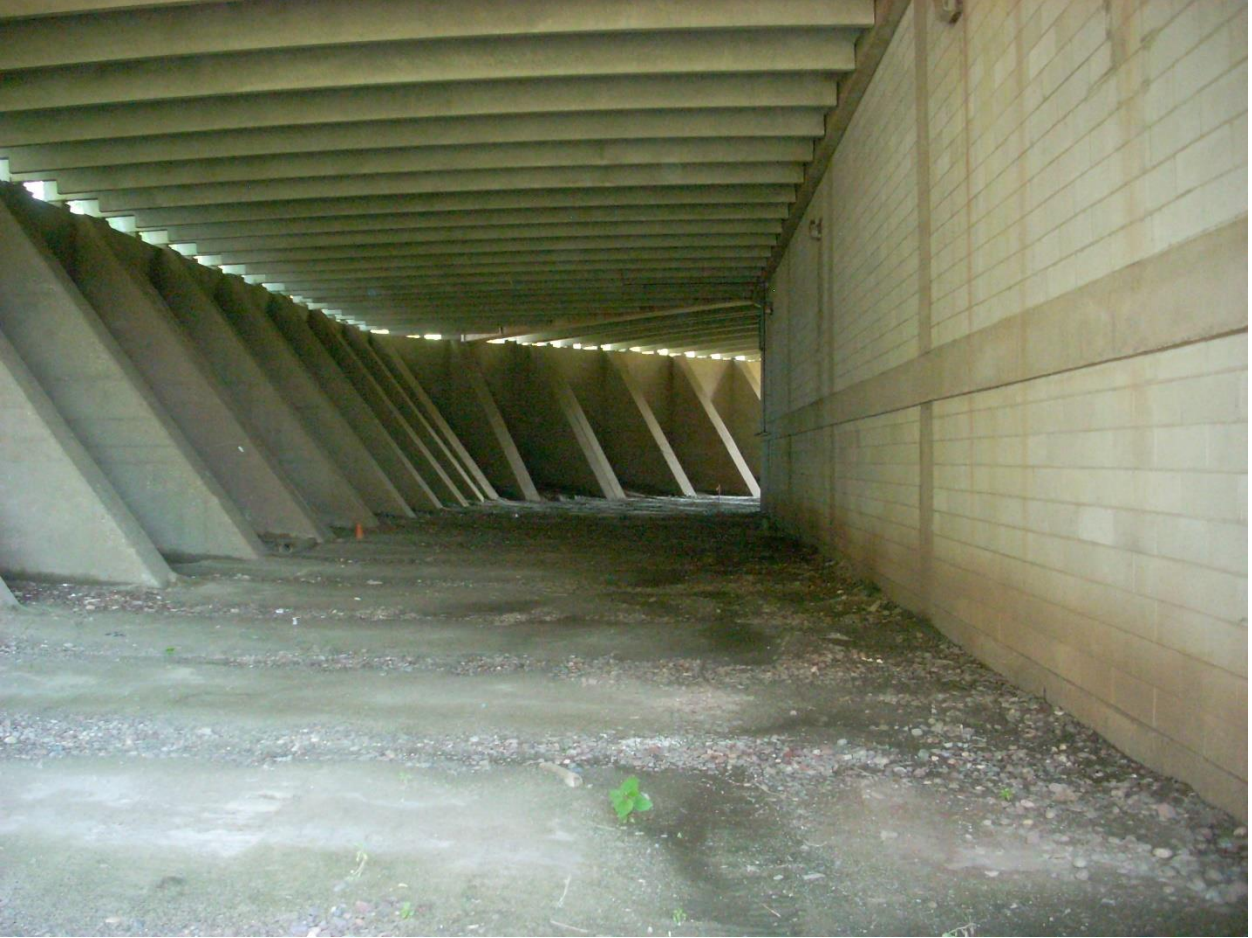
Photo looking North. Toe drain replacement proposed for floodwall toe to right of buttressed concrete floodwall (under Riverpoint Condominium deck).
