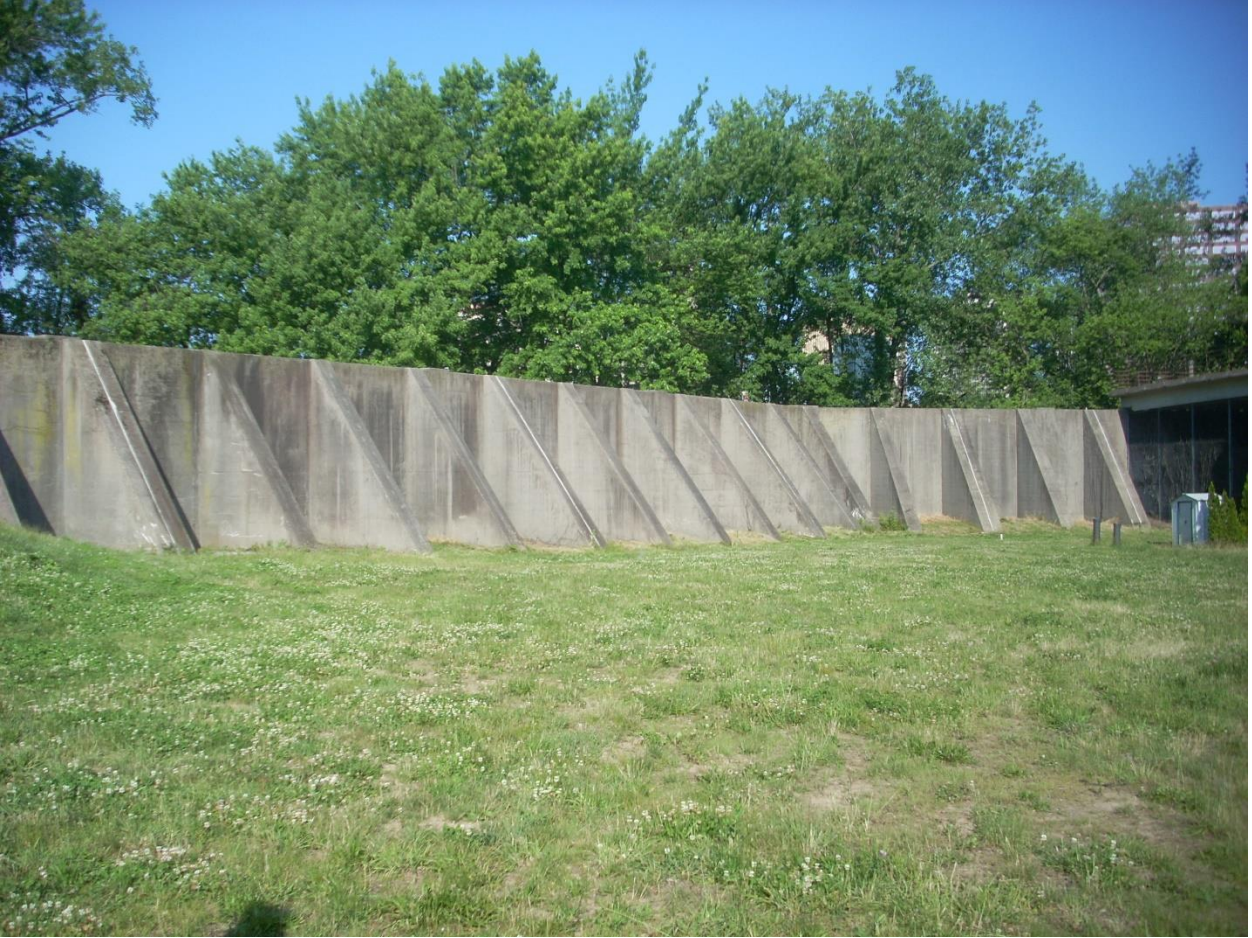
Photo looking North. Toe drain replacement proposed for floodwall toe to right of buttressed concrete floodwall.
