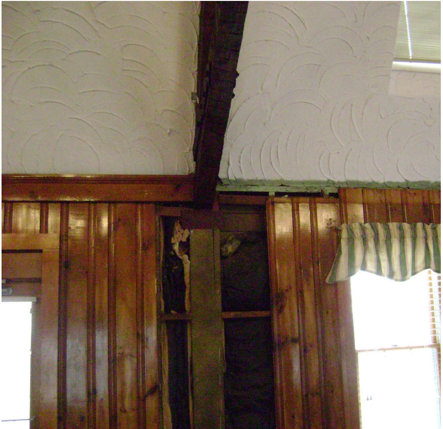
Photo EW1 – North Wing Ballroom (looking towards west) Removed wall paneling to expose truss support column.
