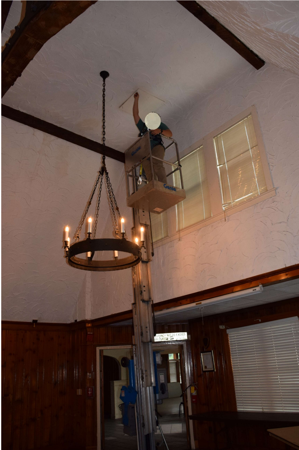
Photo A1 – North Wing Ballroom (looking towards southeast) All attached photos were taken from ceiling access panel.
