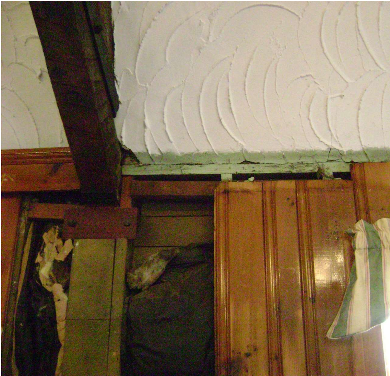
Photo EW2 – North Wing Ballroom (looking towards West) Removed wall paneling to expose truss support column.
