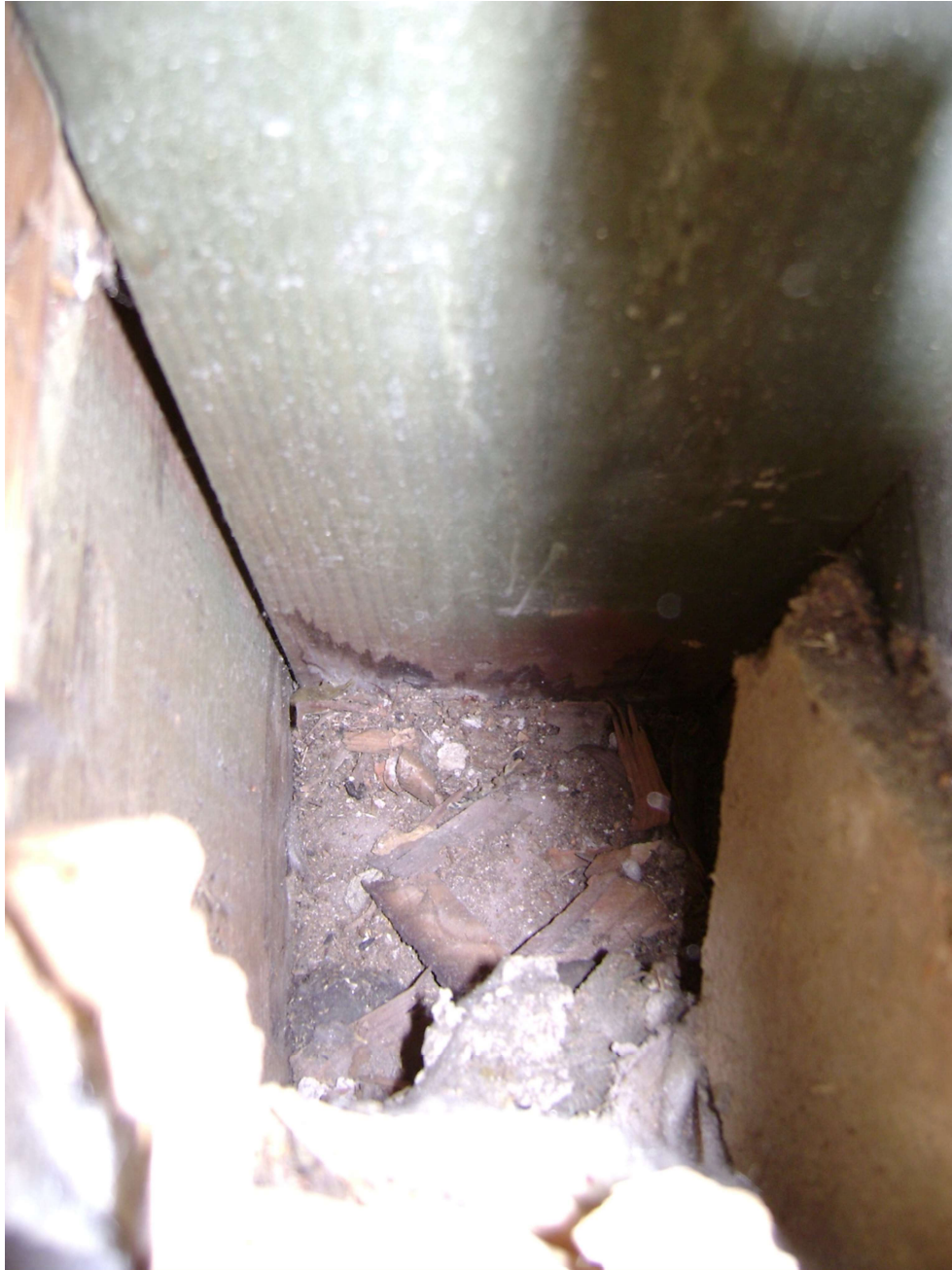
Photo EW8 – North Wing Ballroom Truss support column at base of wall.
