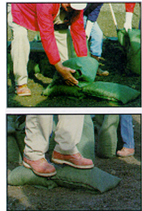
Place each succeeding bag tightly against and partially overlapping the previous one. Compact and shape each bag by walking on it.
