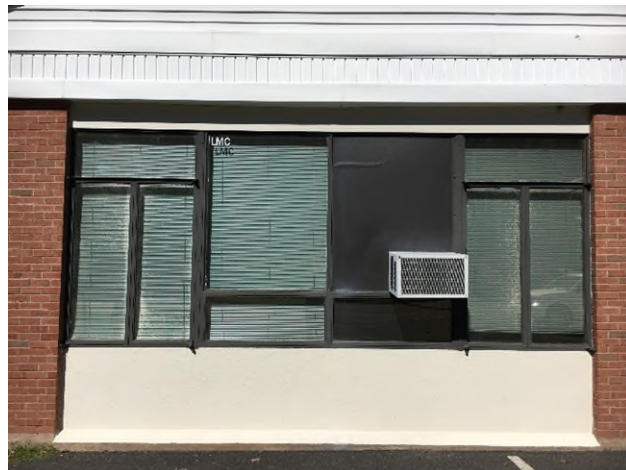
Example of Classroom Ventilation at Pitkin
