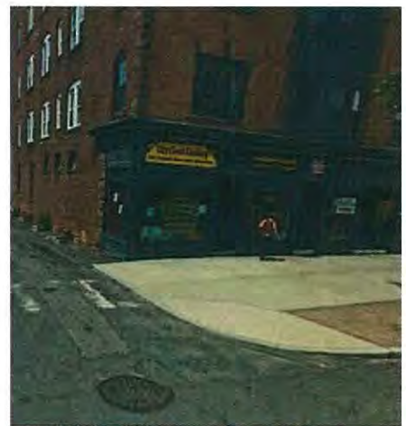
Figure 12. Misaligned Handicap Ramp at Roberts Court
