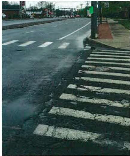
Figure 9. Poor Pavement and Crosswalk Conditions at Willis Street
