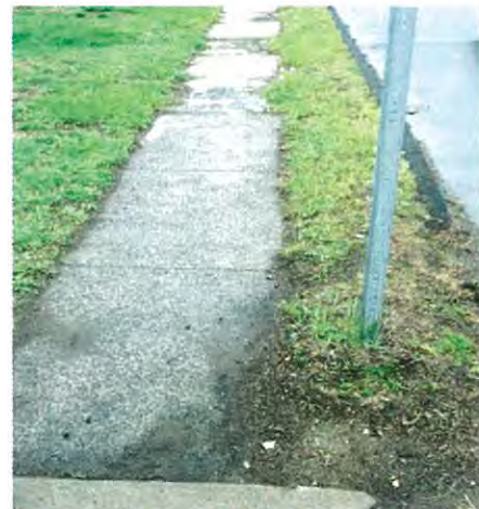
Figure 13. Poor Sidewalk Condition Between the Town Hall Road and Connecticut Blvd
